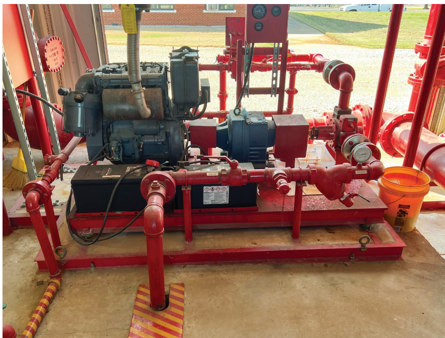
The facility operator agreed to GST's recommendation that PFAS-SOL be deployed to reduce the concentrations of PFAS residues on the fire-fighting system piping and equipment surfaces.
